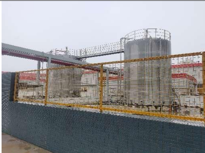
NMP 罐区围堰
